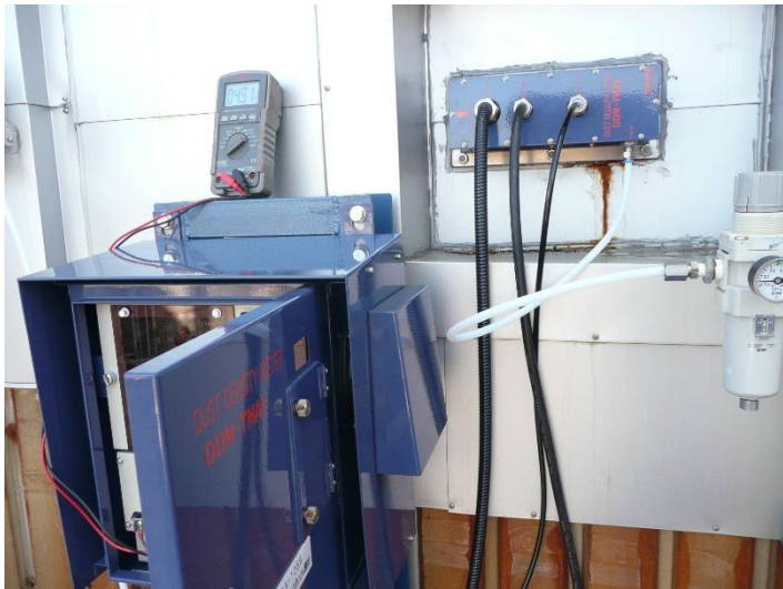
Wiring and piping to DDM-TMA1
